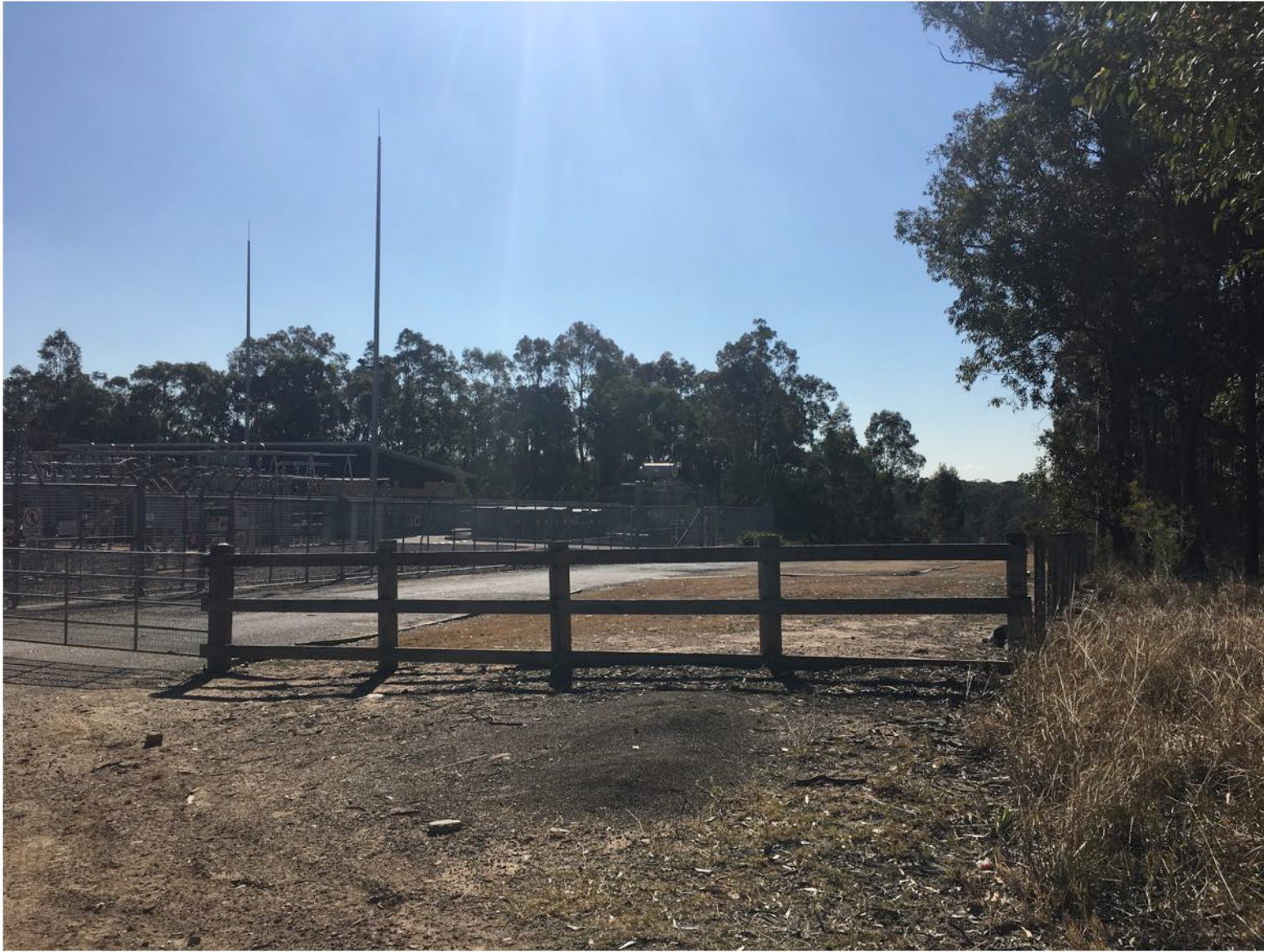
P3 EXISTING ELECTRICAL SUBSTATION
